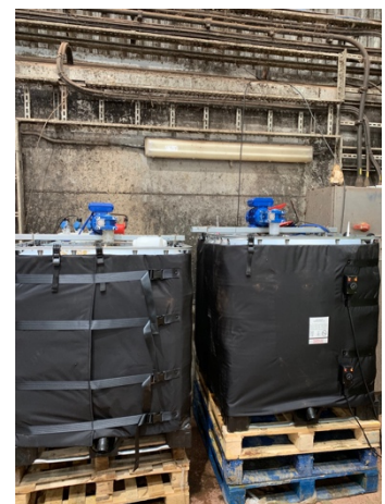
Figure 1 Controlled Batch Reactors in situ
